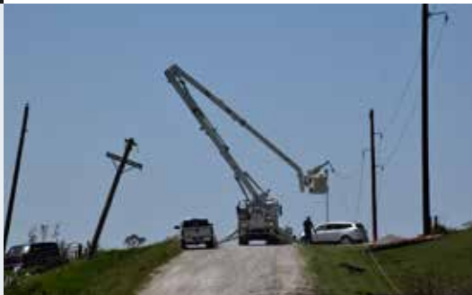
▶ The mid-May storms damaged 109 poles across Central Iowa Power Cooperative's (CIPCO) territory.
